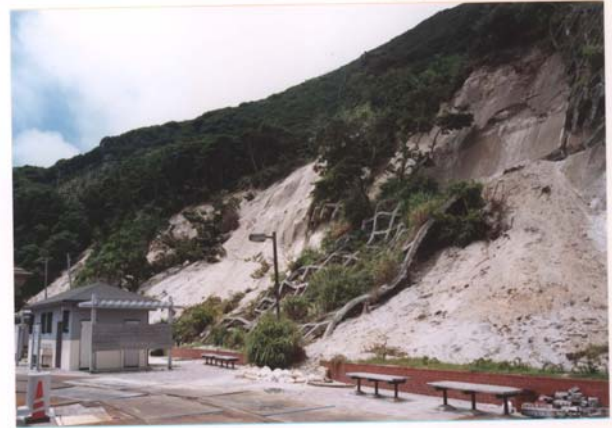
Photo 2 Failure of molded blocks used for slope protection (Miura Harbor)
