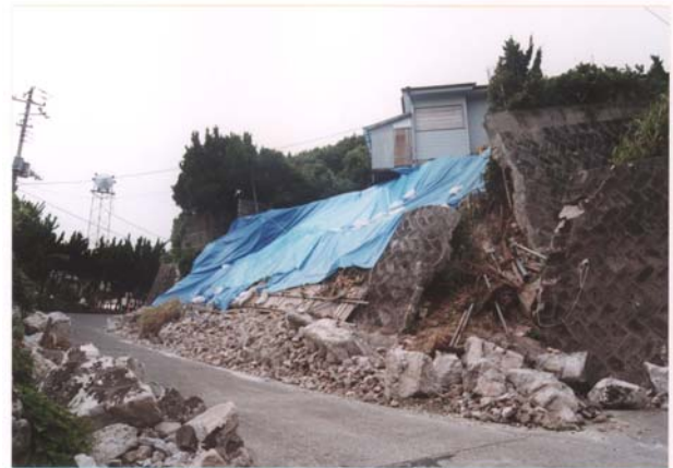
Photo 3 Collapse of a stone masonry retaining wall
