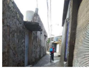
b. Lack of windows that open to the street
