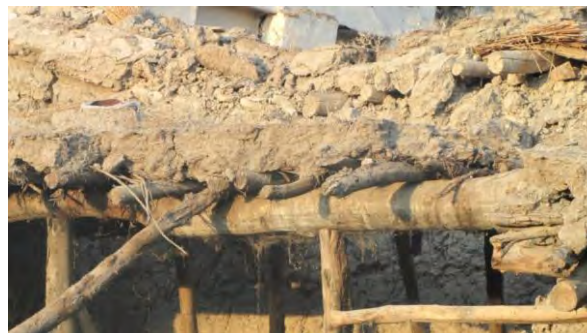
Photo 1.8 Thick layer of mud on the roof.
