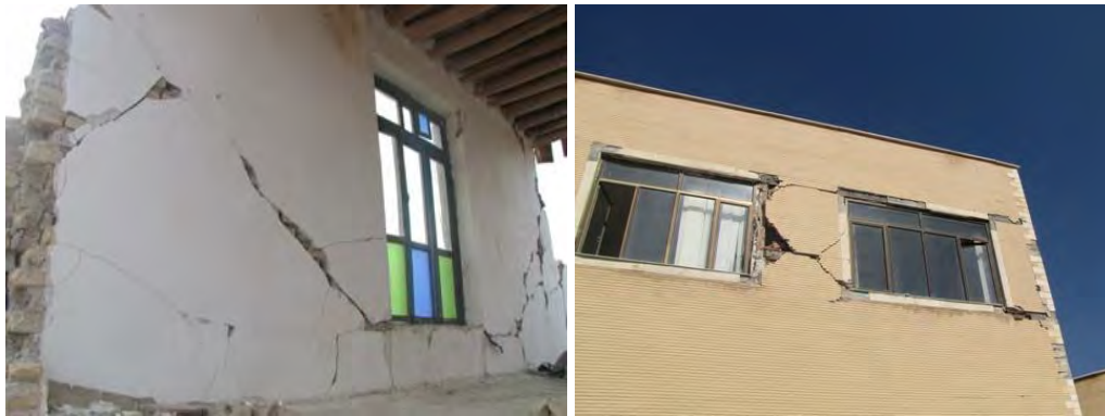
Photo 3.1. Tension diagonal cracks of masonry wall [16, 17].
