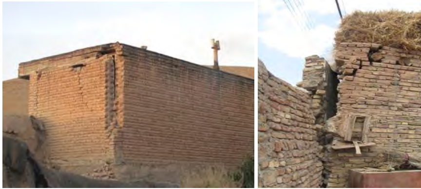
Photo 3.2. Separation of adjacent walls in masonry building.
