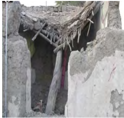
Photo 1.6 Lack of effective connection of the roof to the timbers.
