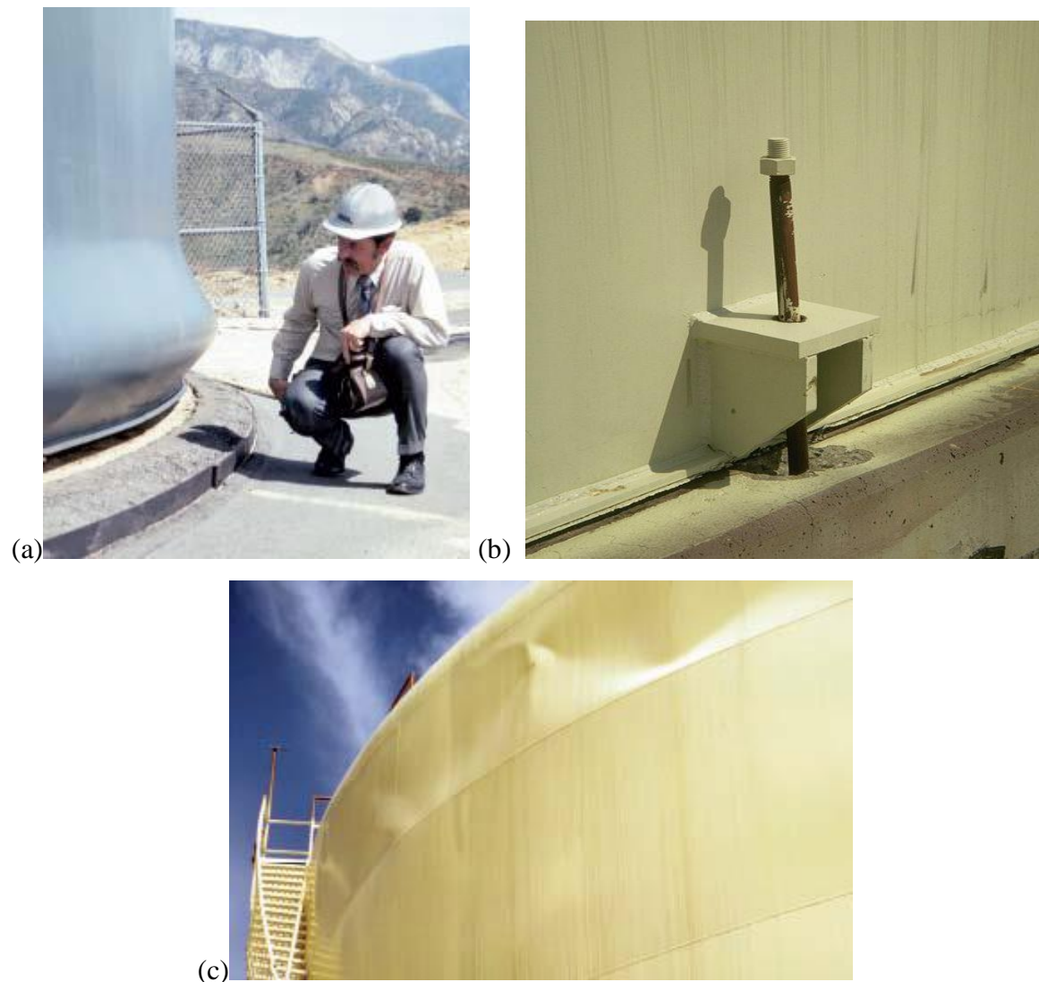
Fig. 1.1. Common damage modes: (a) Elephant-foot buckling, (b) Inelastic stretching of an anchor bolt at the tank base (c) Sloshing damage to the upper shell of the tank (adapted from Malhotra et al. (2000) and Malhotra (2000))
