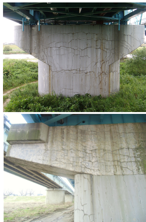
Fig. 1 Typical features of seriously ASR-deteriorated bridge piers.
