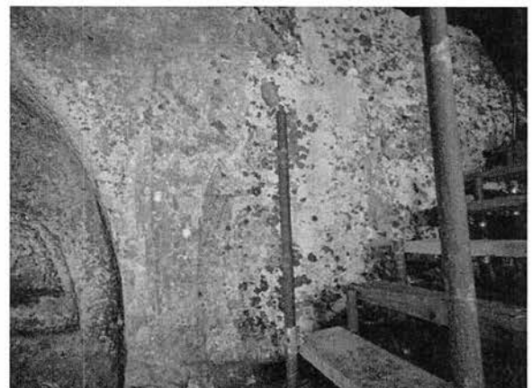
Fig.5 A mural painting deteriorated at the entrance of Saint Nicolas church
