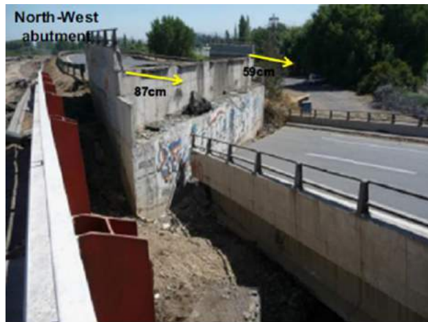
Figure 2.3 Collapse of the Hospital overpass
