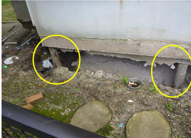
Figure A.19 The pile-supported house which experienced minor inclination in Akitsu town
