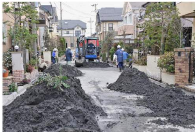
Figure 2.5 Boiled sand on the road in the 2011 Great East Japan earthquake
