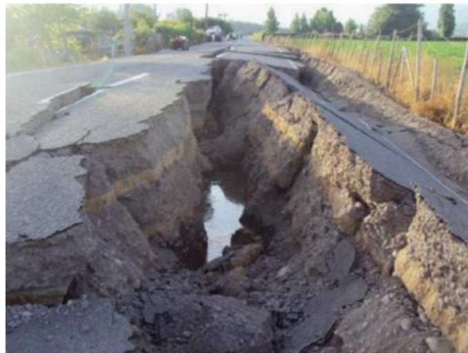
Figure 2.2 Damaged road due to lateral spreading
