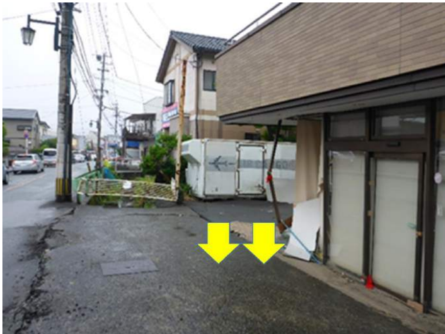
Figure A.8 Liquefaction-induced ground subsidence during the 2016 Kumamoto earthquake
