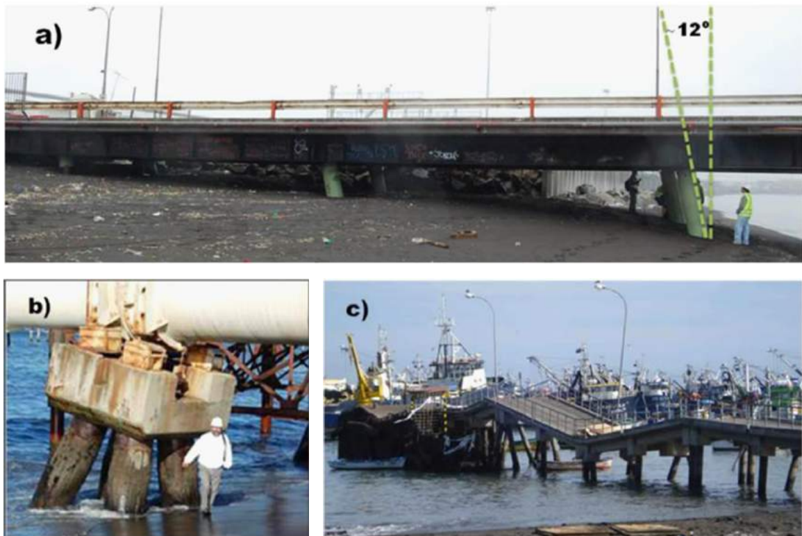
Figure 2.4 Damaged ports due to lateral spreading: (a) Coronel Port, (b) Bocamina Port, (c) Fishermen's Port
