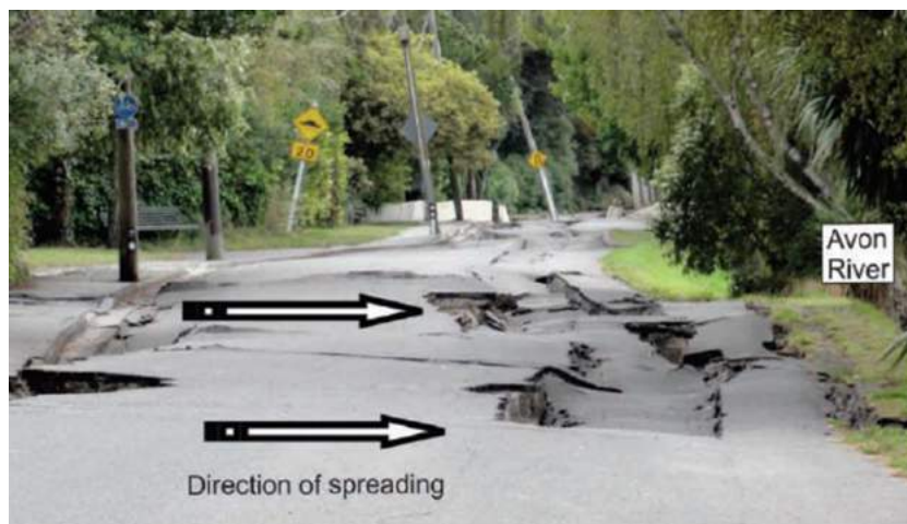
Figure 2.10 Road surface cracks due to lateral spreading towards the Avon River
