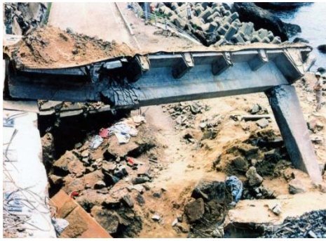
a) Collapse of rock shed
