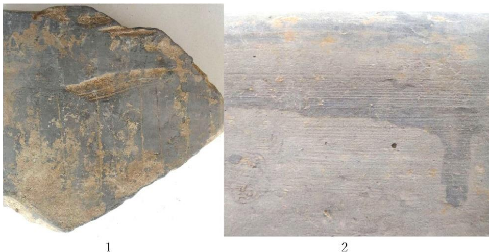
Figure 61 The traces on the convex surface of the roof tiles (Source: Photos by the author) 1. Scraping by plate, 2. Smoothing by fingers
