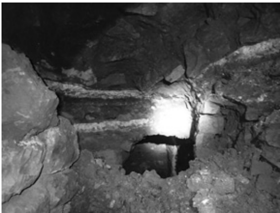
Photograph 5. State of the collapse in tunnel I-27 in September 2017.
