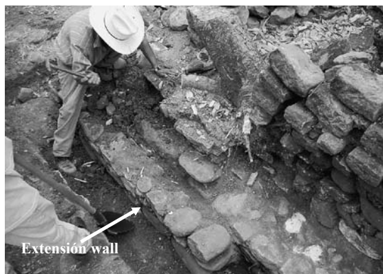
Photo 26: Work done to uncover the underlying foundations of Structure 9L-102-1 st Phase
