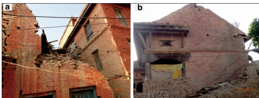
Fig. 16 Damaged buildings with brick structure in Changu village. a Heavily damaged brick building; b cracks in the brick building
