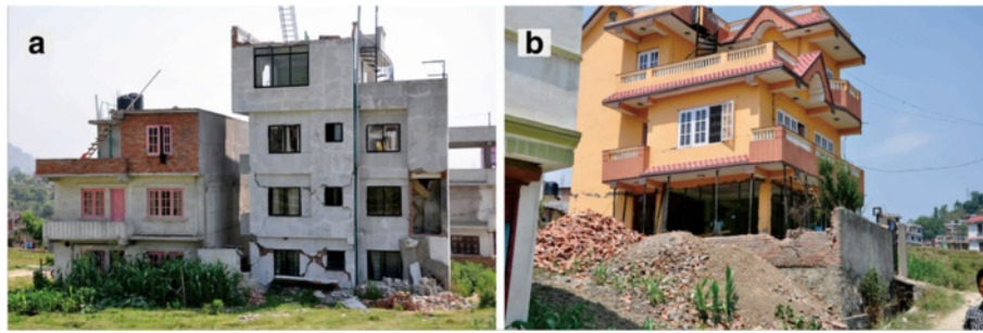
Fig. 23 Damages occurred on the residential buildings in Purano Naikap area. a X-shaped cracks in the first and second floors, some part collapsed; b Collapse occurred to one side of the first floor
