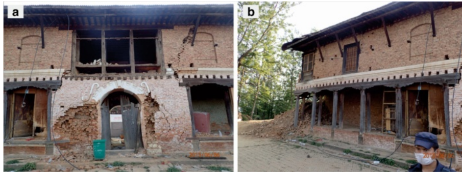
Fig. 17 Damages occurred on the main gate building at the entrance to Changu Narayan. a Collapse around the main gate; b Collapse at the two sides of the gate building
