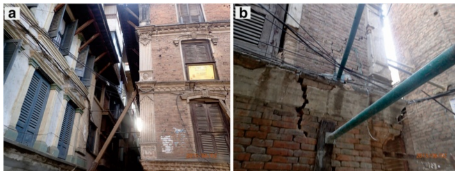
Fig. 8 Heavy damage occurred to the residential buildings in the Durbar Square area. a collapsed buildings supported by wooden sticks; b Cracks in the building and metal supporting sticks
