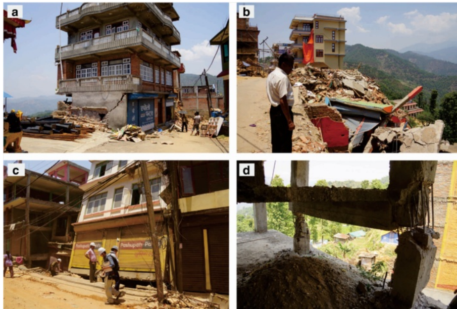
Fig. 13 Partially destroyed or damaged new town area in Chautara. a Cracks in the concrete building; b completely destroyed building; c building tilted to the downslope side; d breakage in pillars of new uncompleted building
