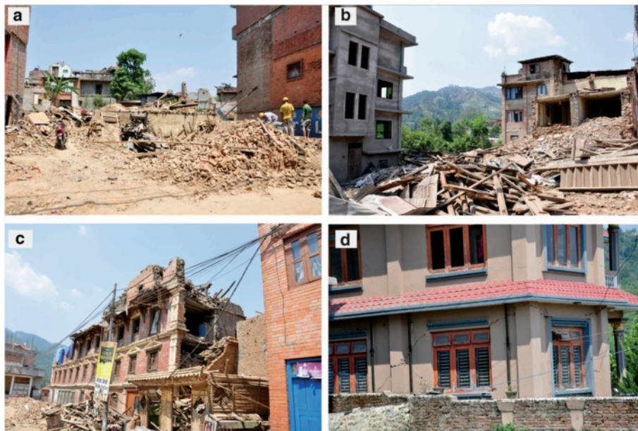
Fig. 18 Building damage situation in Sankhu area. a and b Completely destroyed wooden and brick buildings; c Partial collapses of a three-story building; d X-shapes cracks in a new concrete building
