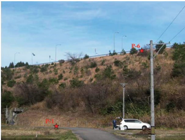
写真-1 西側法面の全景 Photo 1 The panorama of the west side slope.
